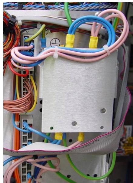
Figure 3 – Completed Filter Installation
