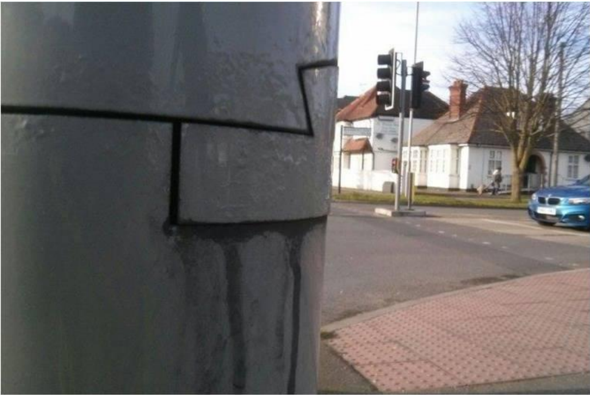
Figure 12 - Black Anaerobic Corrosion
