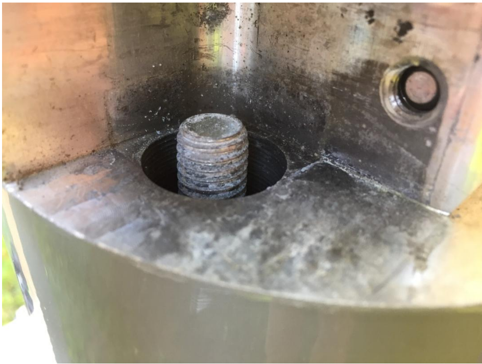
Figure 11 – White Hinge Bolt Corrosion and Incipient Black Anaerobic Corrosion
