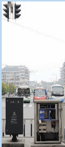
City of Wuhan signal equipment
